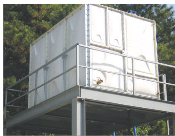
Elevated Type Tank
